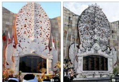
A beautiful memorial for the victims of the tragic Bali bombings has been left to decay, leaning in one crystal clear pool stagnant green, as ornate stone carving covered in mud and one remaining figure barely held together with cracked wire.
